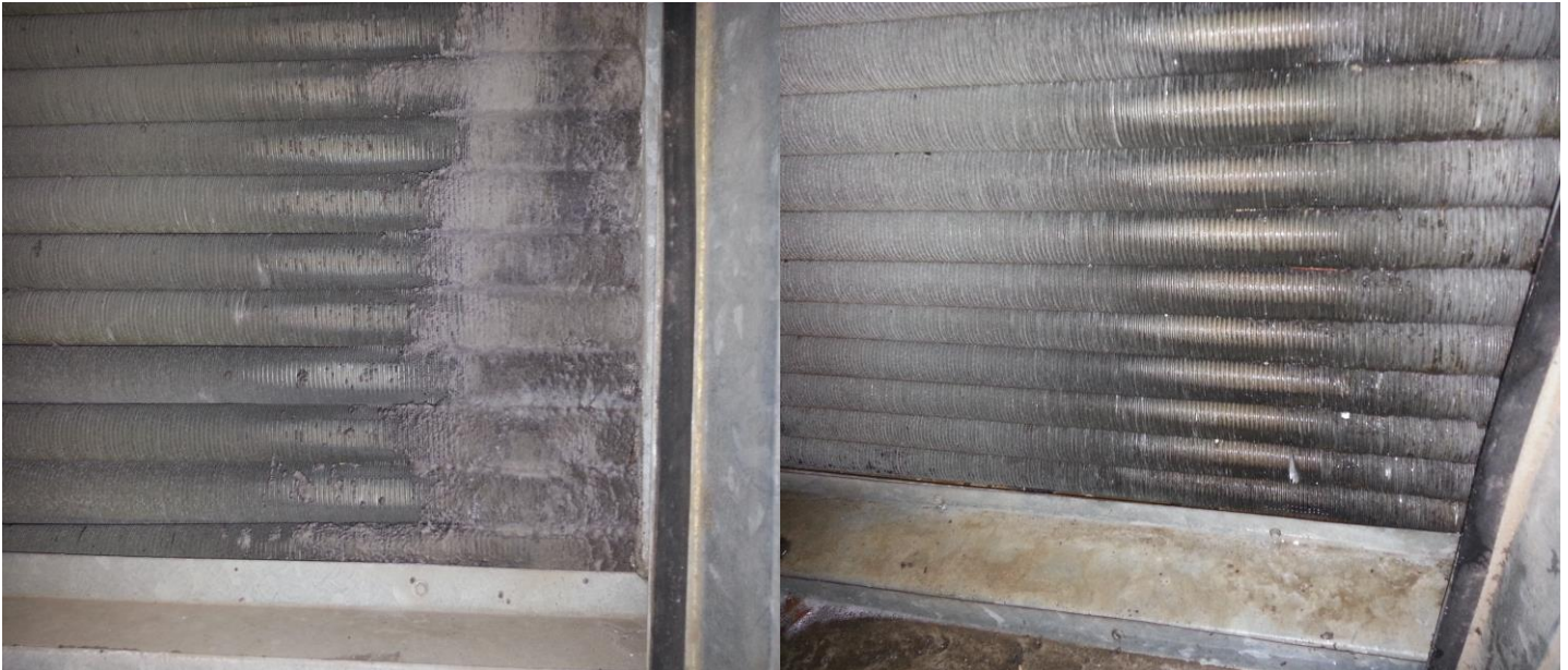
This is a before and after look at one of the Main Air Handlers at [REDACTED]. These are older units with “coin style” coils that are typically very tough to get penetration through the coils. We were able to get penetration through the coils despite the heavy debris.
