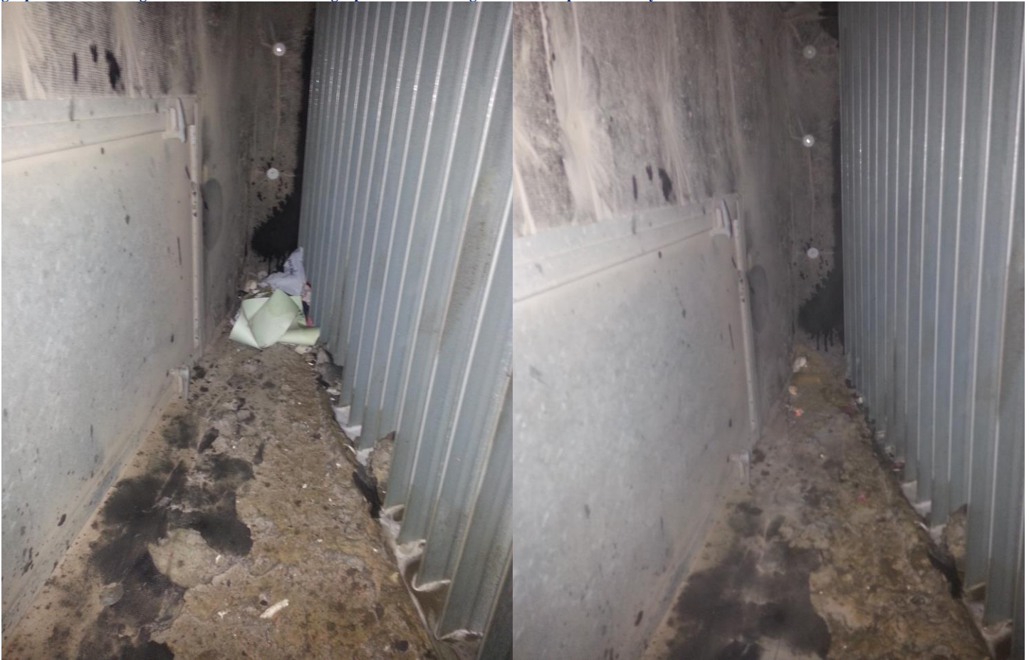
This is a main AHU at [REDACTED] with a bunch of accumulated debris that we cleaned out of the unit before cleaning the coils. The brown is old insulation.
