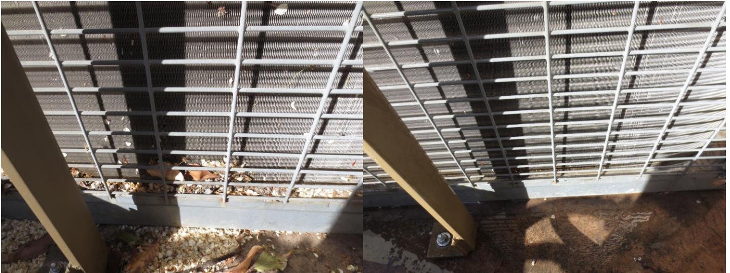
Above is a before and after look at a condenser unit that had a tremendous amount of leaves and debris all over the units restricting airflow.
